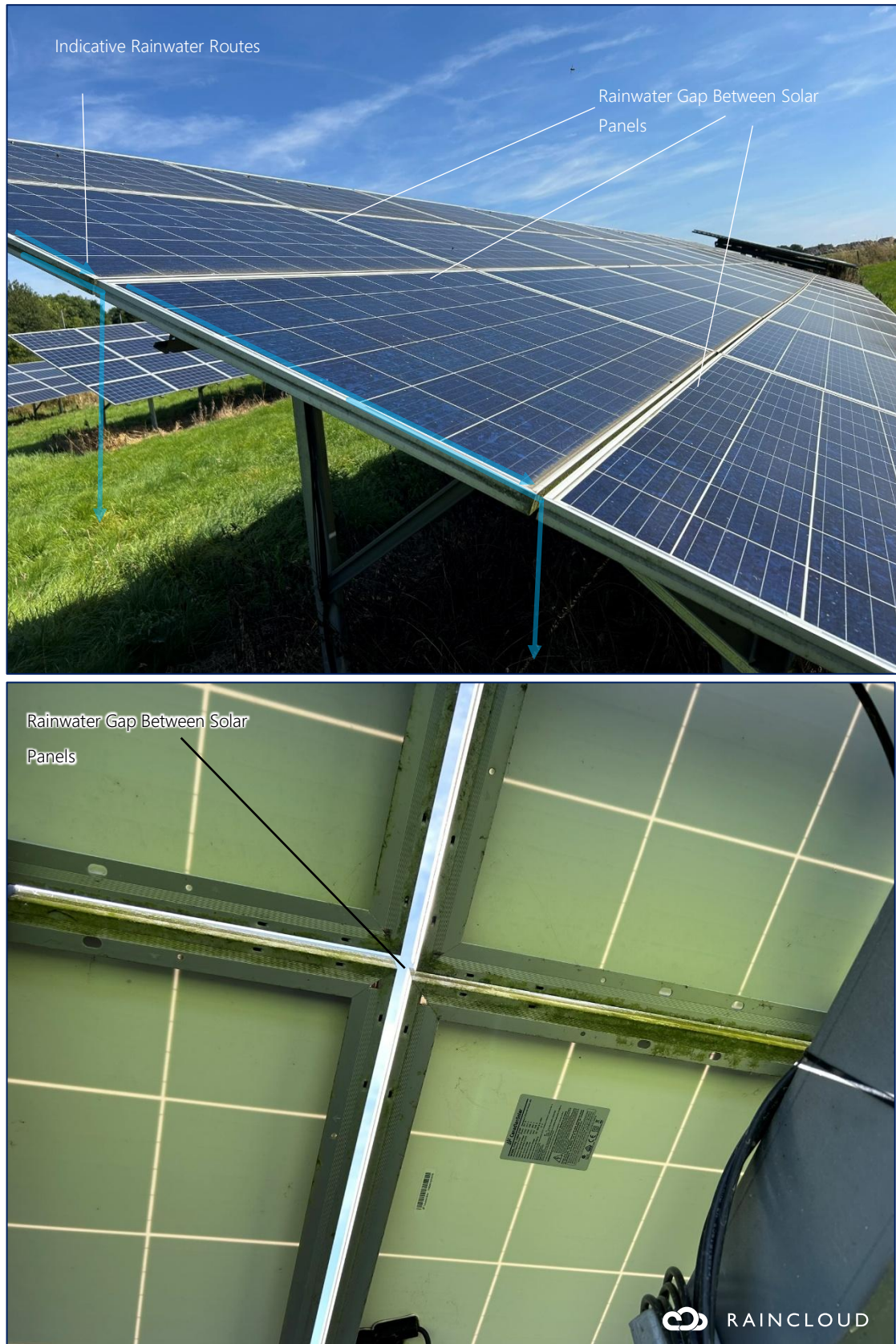
Plate 12-25 Rainwater gaps on PV array table
